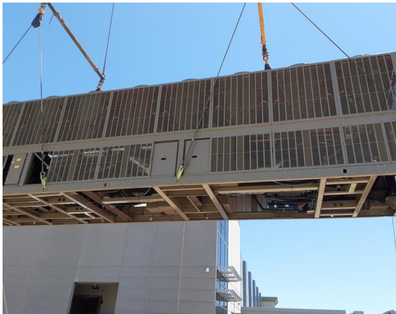
Follett, YORK screw pump chiller with glycol cooling
