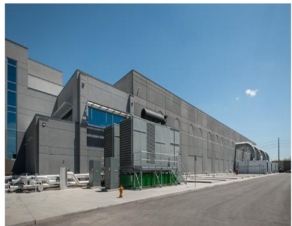
Rolls Royce Deisel generator on top of green fuel tank at CyrusOne in Chandler, AZ
