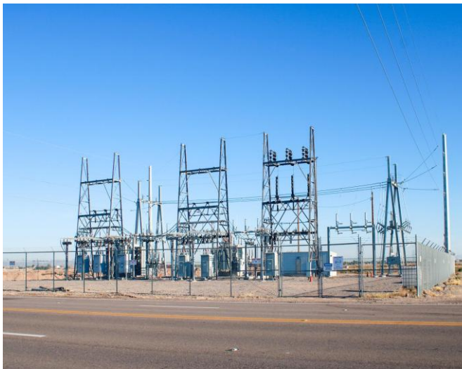
By: ED3 Sonny Dunn Substation, Maricopa AZ
