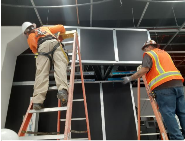
Follett: Assembling the head piece to a CRAH unit inside a data hall at CyrusOne Chandler, Arizona.
