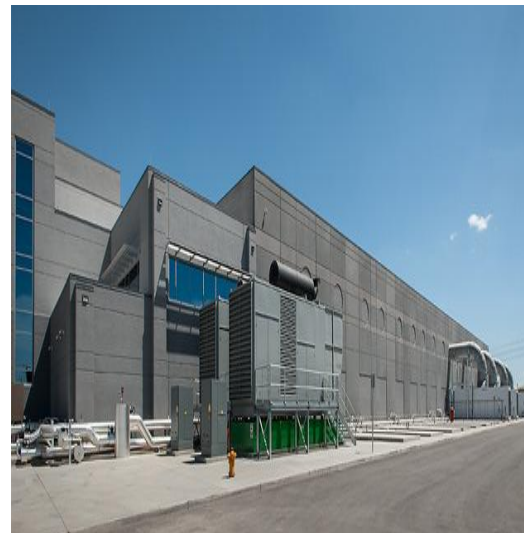
Rolls Royce Deisel generator on top of green fuel tank at CyrusOne in Chandler, AZ
