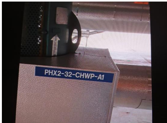
Follett: 500 hp Horizontal chiller pump running backwards with 14 psi suction energy at CyrusOne in Chandler: See Video
